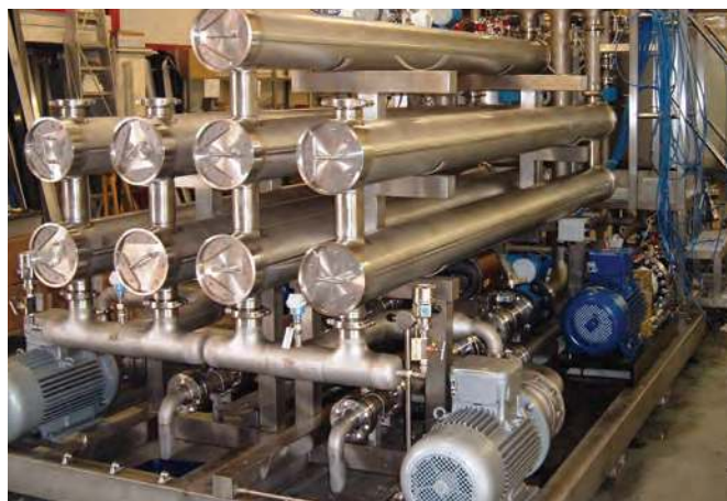
Hydra-Cell pumping for waste stream reduction and salt solution concentration at a pharmaceutical chemical plant.
