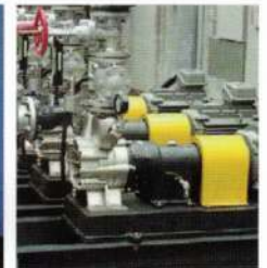
KTM Installed in parallel system
