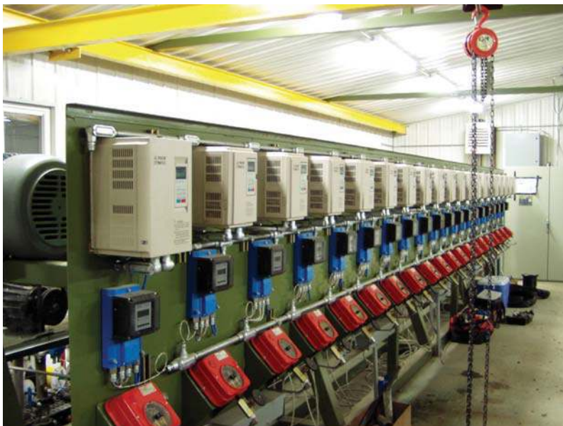
Figure 2. Each pump serves a separate oil well. Pump flow and pressure are regulated via VFD speed control in response to conditions in the well.
