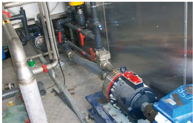
RO treatment of high TDS groundwater at a cement production plant.
