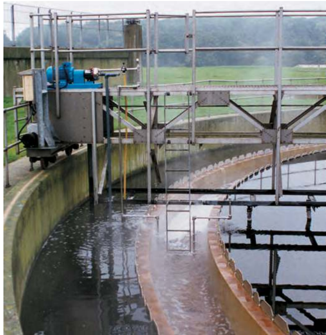
Hydra-Cell operating in a wastewater treatment facility.
