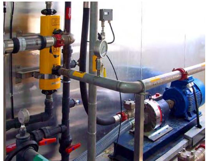
RO recovery device.
