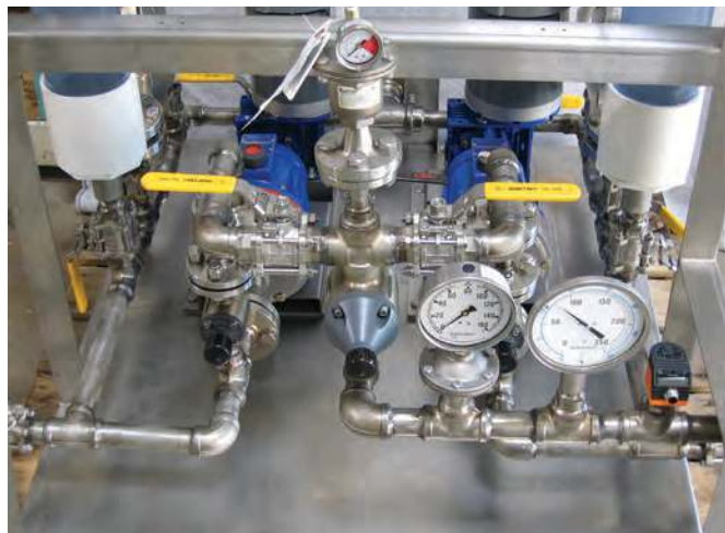
Metering flocculants for wastewater treatment.
